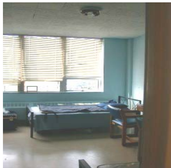
Typical double room with worn-out interior and furnishings, no A/C, Wamack Residence Hall
