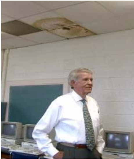
C.C. Cameron inspects ceiling leaks over computer stations in Lester Hall
