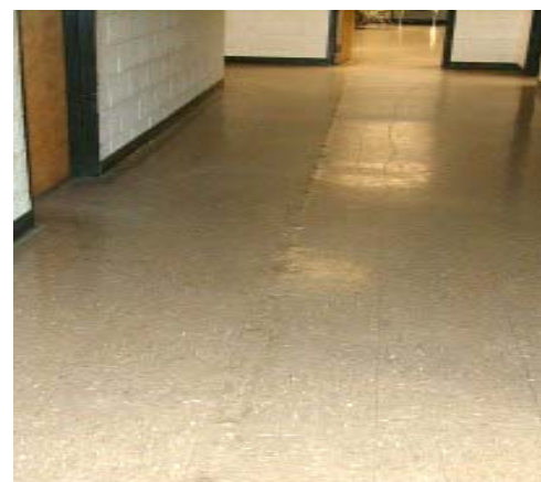
Vinyl tile flooring needs replacement
