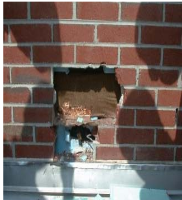
Test hole to determine leak source, at time of Campus Visit. The problem has since been resolved, Jenkins Science Complex
